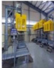
Gas Bottling Unit
